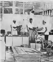
WHILE SOME workers uncrated and moved in furniture, other Mechanical men worked on lighting fixtures, above. Room panel dividers were installed by Mechanical-Carpenter employees.
